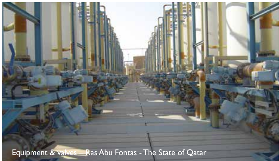
Treatment plant (Limestone Filters) – Ras Abu Fontas - The State of Qatar
